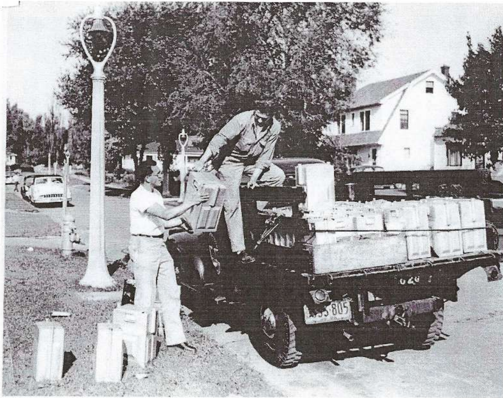
Rochester Gas & Electric crew delivering new gas meters to houses in Roselawn, Meadowbrook, and Bel-Air.
